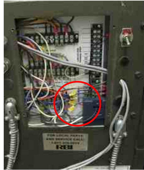
Figure 13. Current switch to monitor runtime of the pump between the DHW boiler and the tanks
