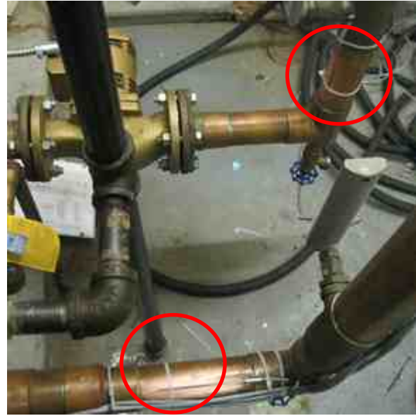
Figure 16. Boiler input and output T sensors
