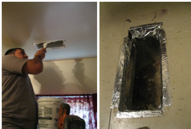
Figure 5. Applying mastic to ceiling register boot (left) and register boot sealed to floor with foil tape
