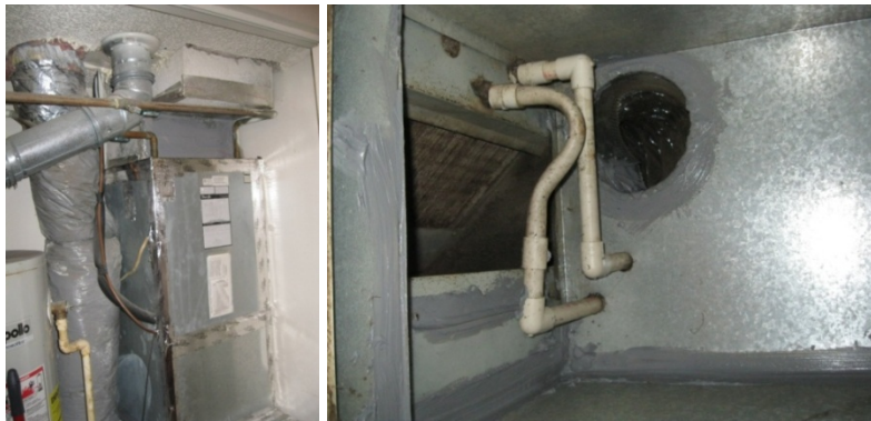
Figure 7. Air handler sealed with foil tape (left) and return plenum sealed with mastic (right)
