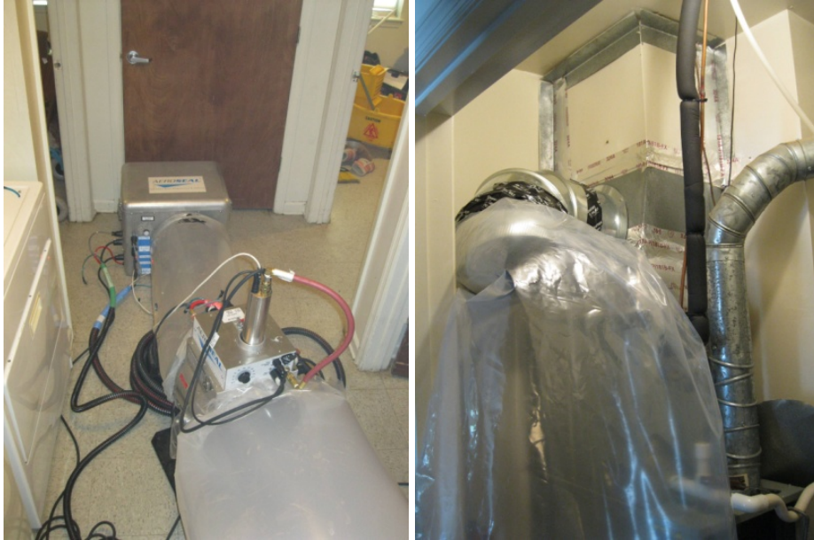
Figure 8. Aroseal equipment (left) connected to supply plenum (right)
