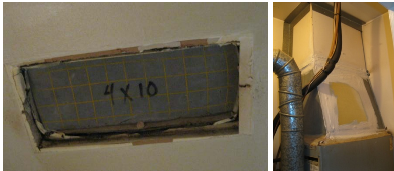
Figure 9. Register plugged during Aroseal process, showing gaps that must be hand-sealed (left); supply plenum repaired after Aroseal process (right)
