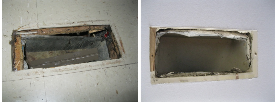
Figure 3. Register boot pulling away from floor (left) and ceiling (right)
