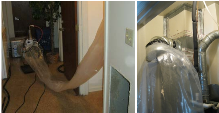
The Assembled injection system includes a blower/heater (background) and the sealant injection unit (foreground)
