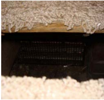
Figure 5. Before: Disconnected duct boot behind floor register
