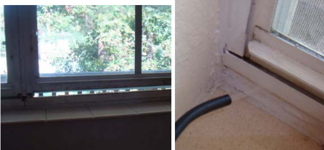
Figure 15. Before: Old windows not closing tightly
