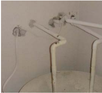
Figure 19. Before: Openings around water heater pipe penetrations
