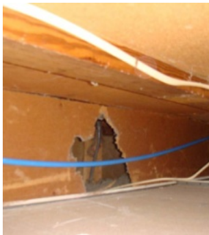
Figure 9. Before: Opening in wall above dropped ceiling
