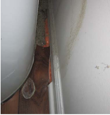
Figure 25. After: Crack under wall in mechanical space sealed to floor with foam
