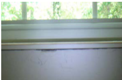
Figure 13. Before: Gaps around window sill resulting from poor installation of windows
