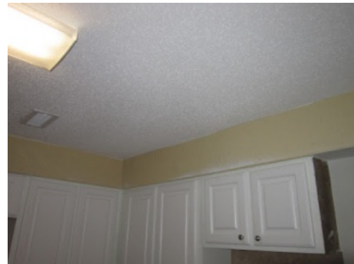
Figure 8. After: New gypsum board ceiling in kitchen isolates wall penetrations from living space
