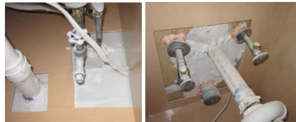
Figure 18. After: Plumbing penetrations sealed around pipes and behind escutcheons with foam and caulk
