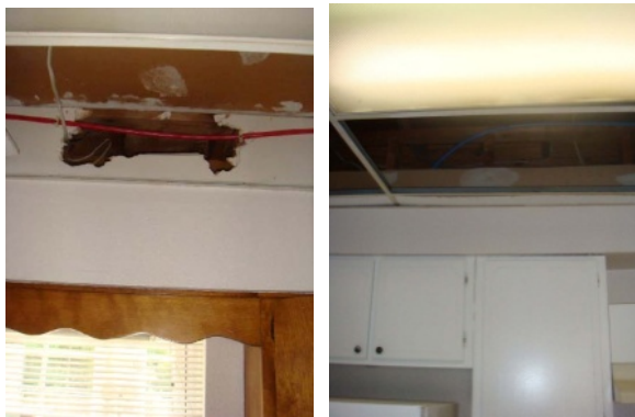
Figure 7. Before: Openings in walls above dropped ceiling in kitchen
