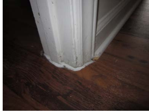
Figure 26. After: Crack at bottom of door jamb sealed to floor with caulk
