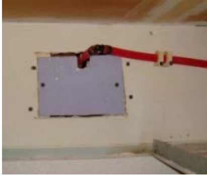
Figure 11. Before: Poorly patched plumbing opening in wall above dropped ceiling
