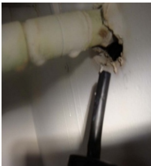
Figure 17. Before: Opening in wall around pipe being tested with smoke stick reveals air pathway
