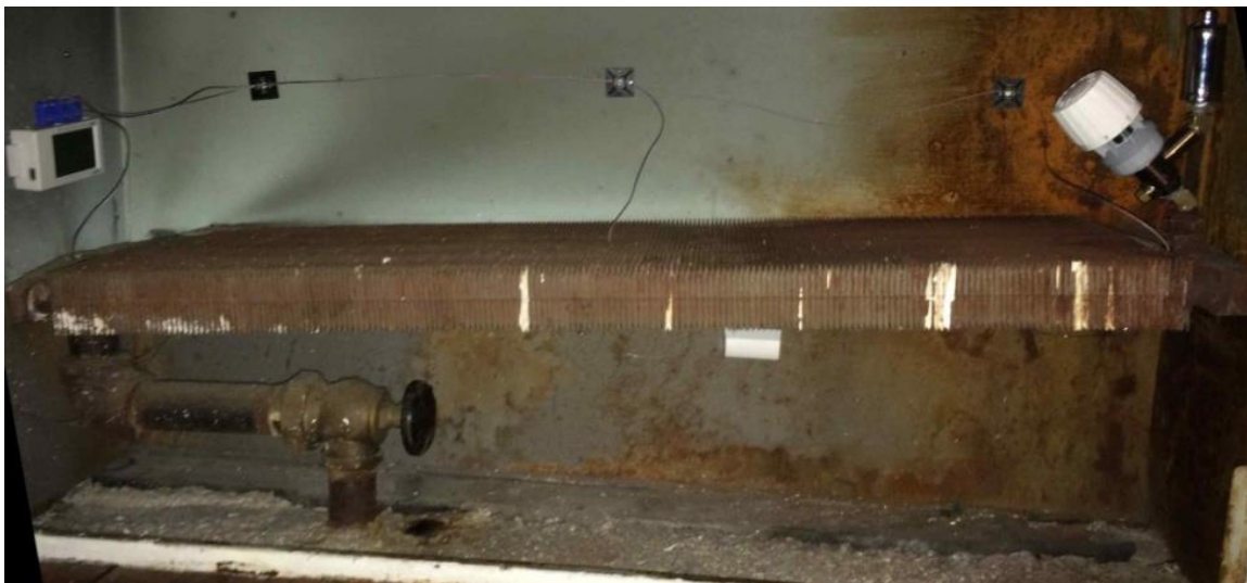
Figure 3. Typical convector with datalogger, thermocouples, and TRV installed
